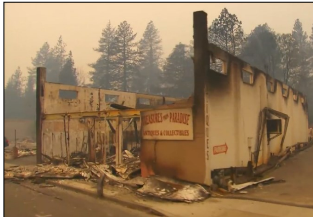
Fire damage of a business in Paradise, CA ( link ).
