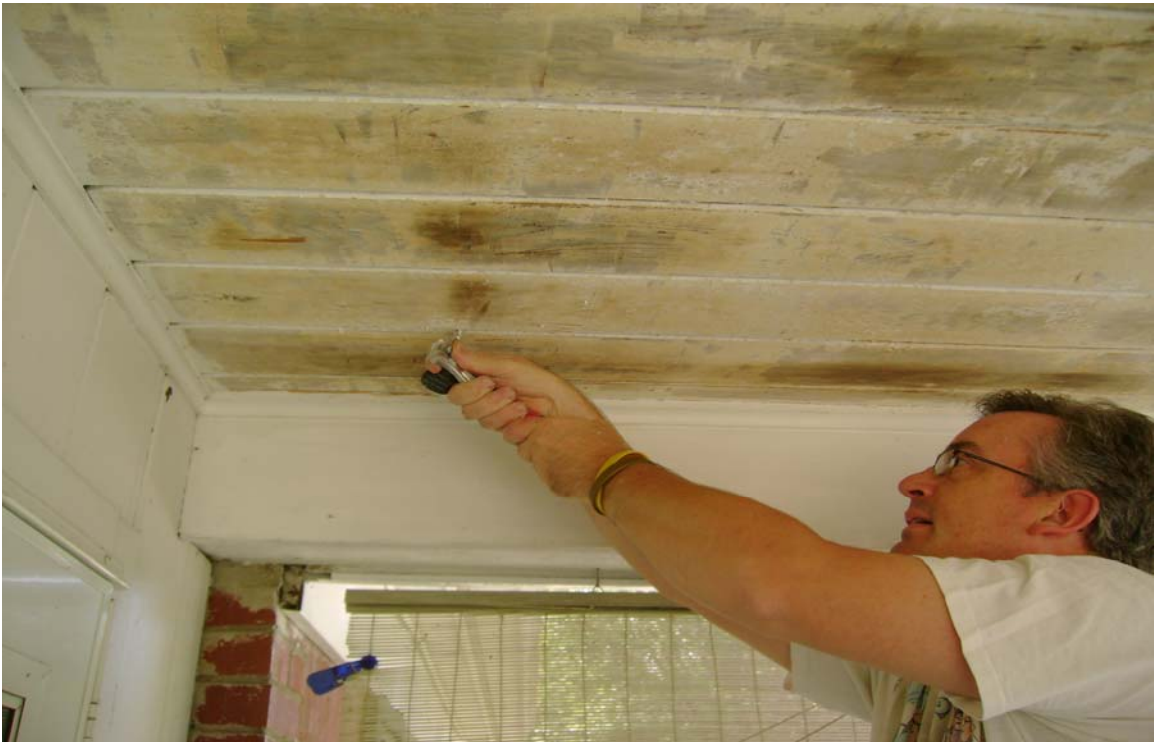
Step #4 Removing the remaining paint in the v-groove of the ceiling boards using a carbide blade pull-back paint removing tool. Notice slight surface charring which is easily removed with light sanding.
