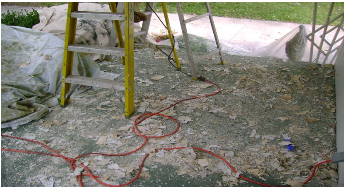
Porch floor showing removed paint from the ceiling
